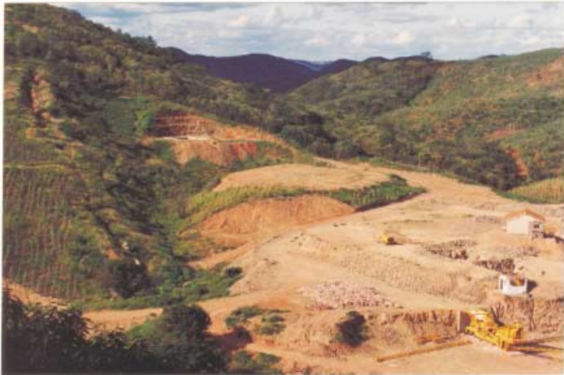
Figure 3.12 View of the Cachoeira de Minas mine. Gold is recovered by cyanide heap leaching .
