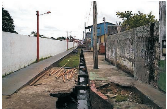
Figure 4 – Open sewage channel near the public water wells at the Paraiba pumping station.
