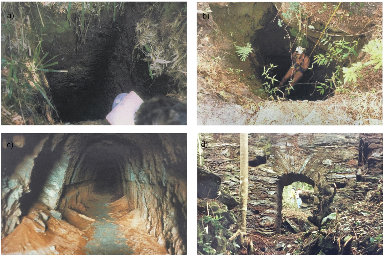
Fig. 16. (a) Shaft No.10 of rectangular shape and depth of 8.5 m. (b) Shaft No.13 of circular shape with 17 m depth. (c) Arched gallery. (d) Stone arch. Photos compiled from IEPHA-MG (1998).
